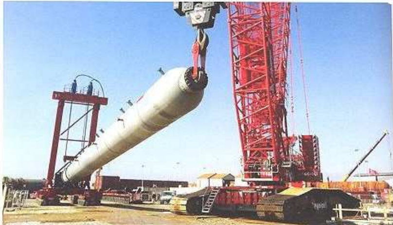
Two reactors were transported, lifted and installed in a refinery in the north of Italy by Fagioli in March. Each reactor was more than 45 m long, with a net weight of almost 400 tonnes. Fagioli used 30-axle line SPMTs to move the reactors, then a crawler crane LR1750 with a capacity up to 750 tonnes, and a tailor-made tailing frame structure positioned on 2 x 10-axle line SPMTs, with two L600 strand jacks on top of the structure used to perform the tailing operations.
